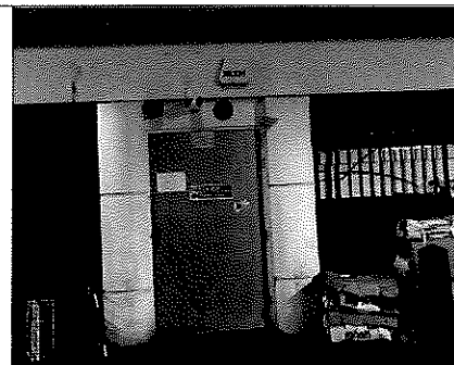
No notice at rear of building re noise of bottling.
